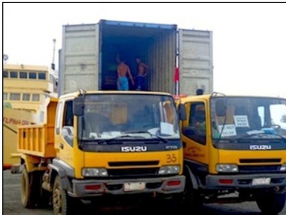
The construction materials being transferred from the container van to four trucks of the Iloilo provincial government
